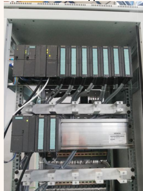
Power Supplies PLC
